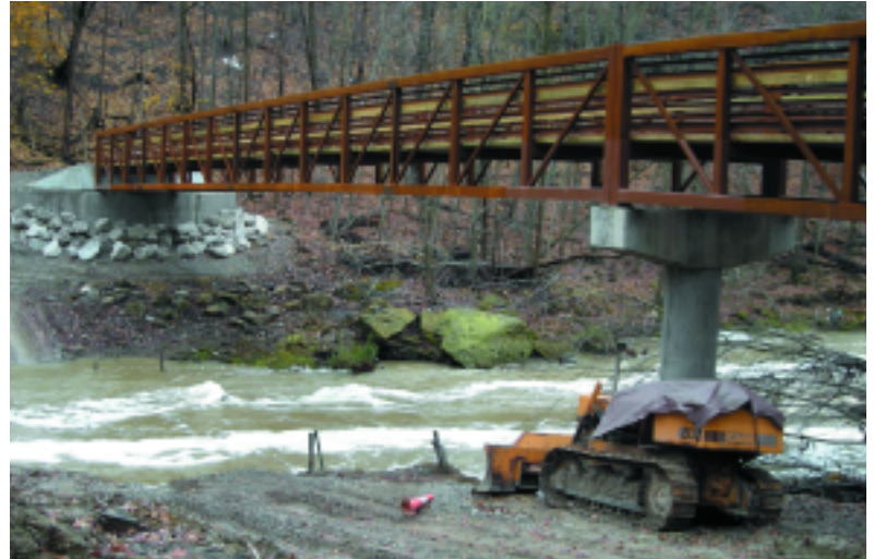
The new pedestrian bridge over the west branch of the Black River is in place in Elyria. The West Falls and the Lake Avenue Bridge can be seen in the background.
